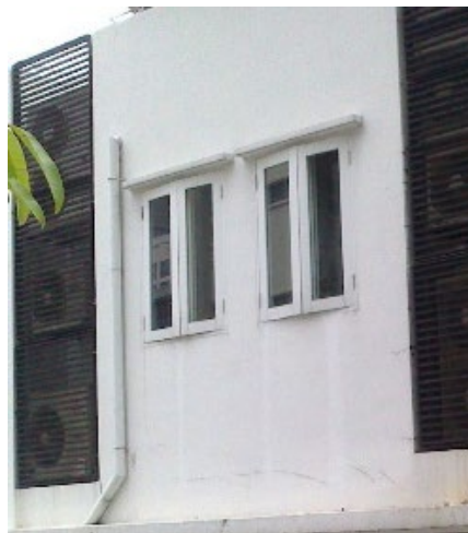
A/C ledges: Louvers with insufficient depth
