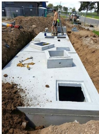
Detention tank with multiple access hatches
