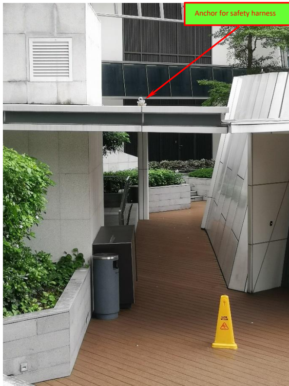
Canopy with anchor for safety harness
